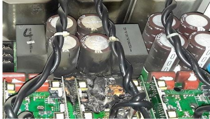
Figure 2. Damaged inverter from a change in electric quality
